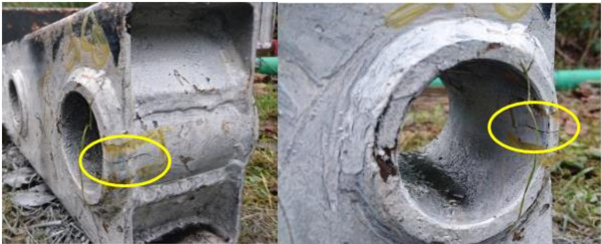
A-Frame pin circular bore cracking. (visual & mpi)
