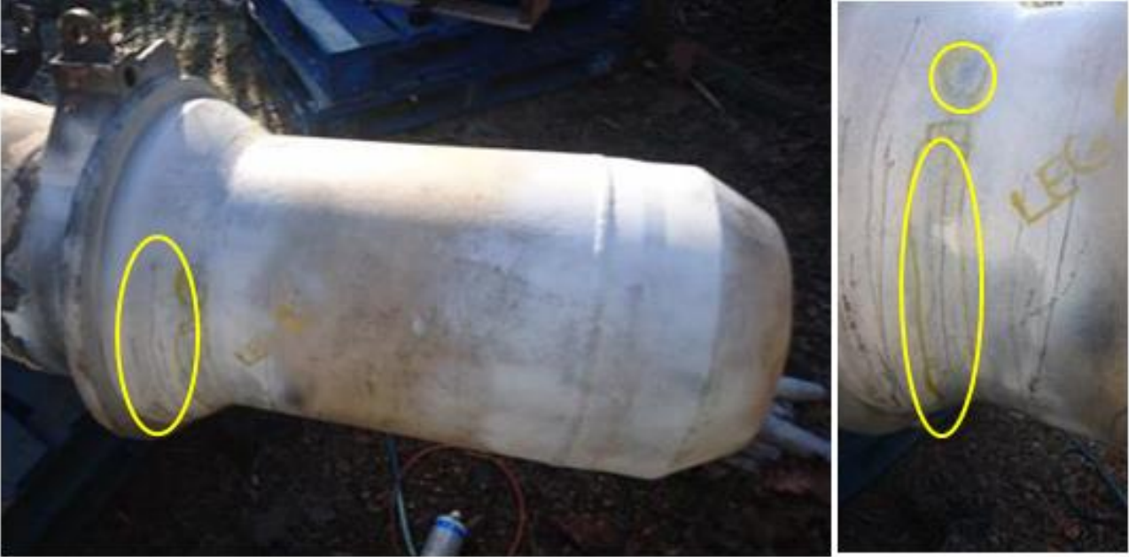
Main leg spigot cracking (visual, mpi & UT)
