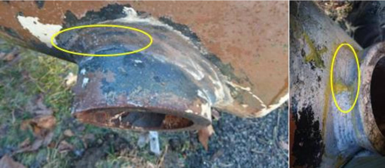
Lower support leg bore circ welds cracking (visual & mpi)
