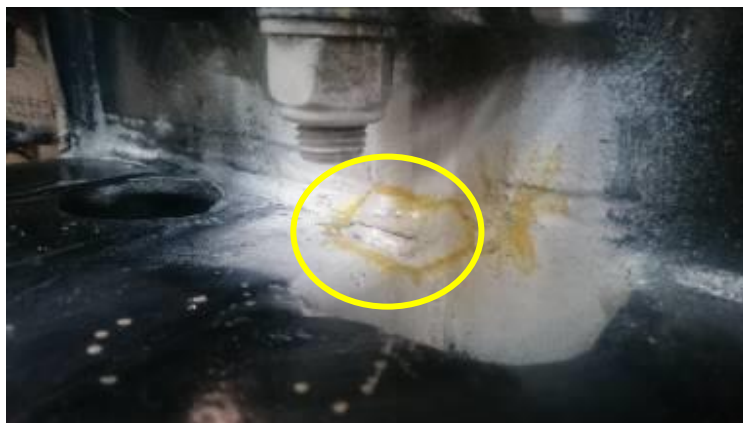
Strengthening gusset cracking below seat
