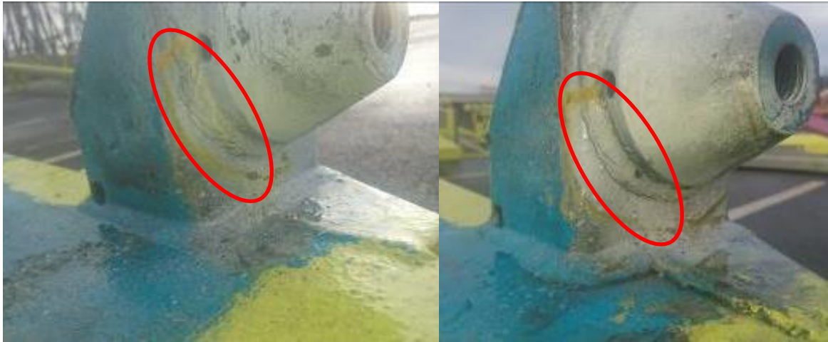
Reverchon Crazy Mouse support column track allocation cone cracking
